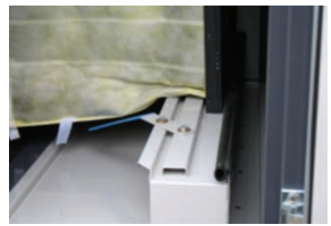
The DanX filter section is designed for high humidity and a chlorinated atmosphere.
