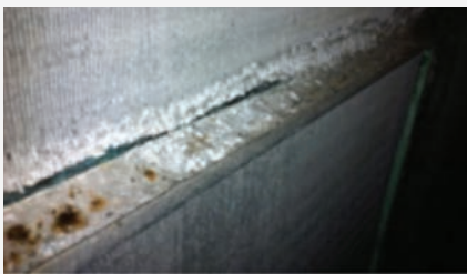
Unprotected heating coil fins were badly corroded after just 10 years.
