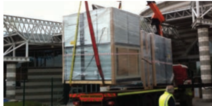
The DanX air handling units arrived with the solution agreed and Dantherm Engineer's set to work:
