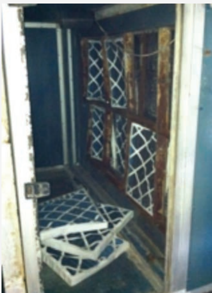
Filters were an ineffective, low grade specification, with cardboard frames that collapse in a moist environment
