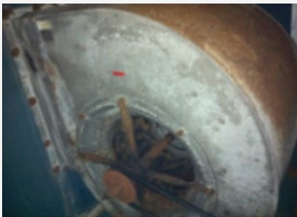
The existing belt drive fans were unpainted and corroded in the chlorinated atmosphere
